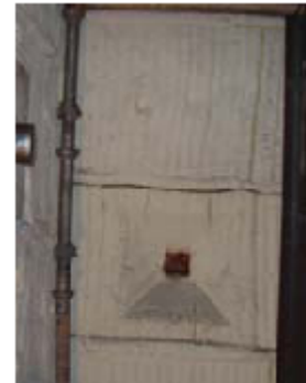
Figure 3 – Uncoated Z-Blok® after 3 months in service.
