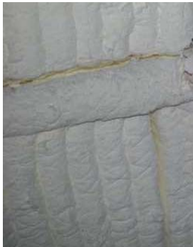
Figure 1 – Emisshield® coated Z-Blok® before start up.
